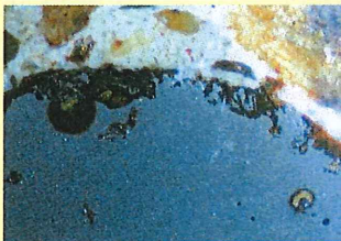
37 MAGNIFICATION CORROSION AND DIFFUSION OF IRONOXYDE HYDRATES THROUGH THE CONCRETE POROSITY
